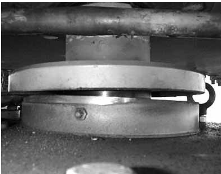
Figure 4. Canted Output Shaft Due to Upper Output Shaft Bearing Failure.
