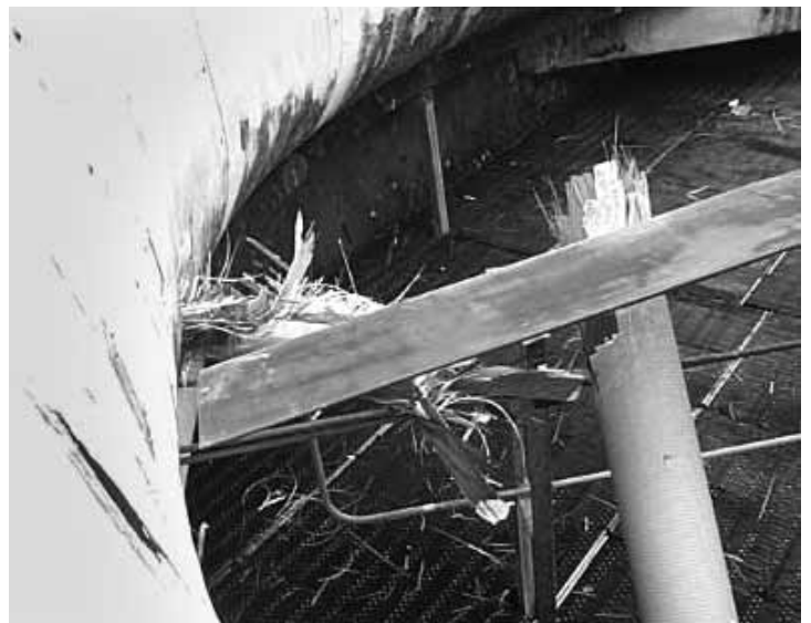
Figure 4. Collateral Damage to Fiberglass Motor Shaft and Fan Blades.
